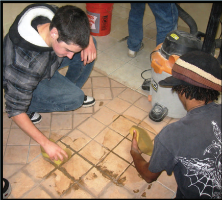
Neal Bentley and Andre Williams grouting tile in a new Habitat for Humanity office
